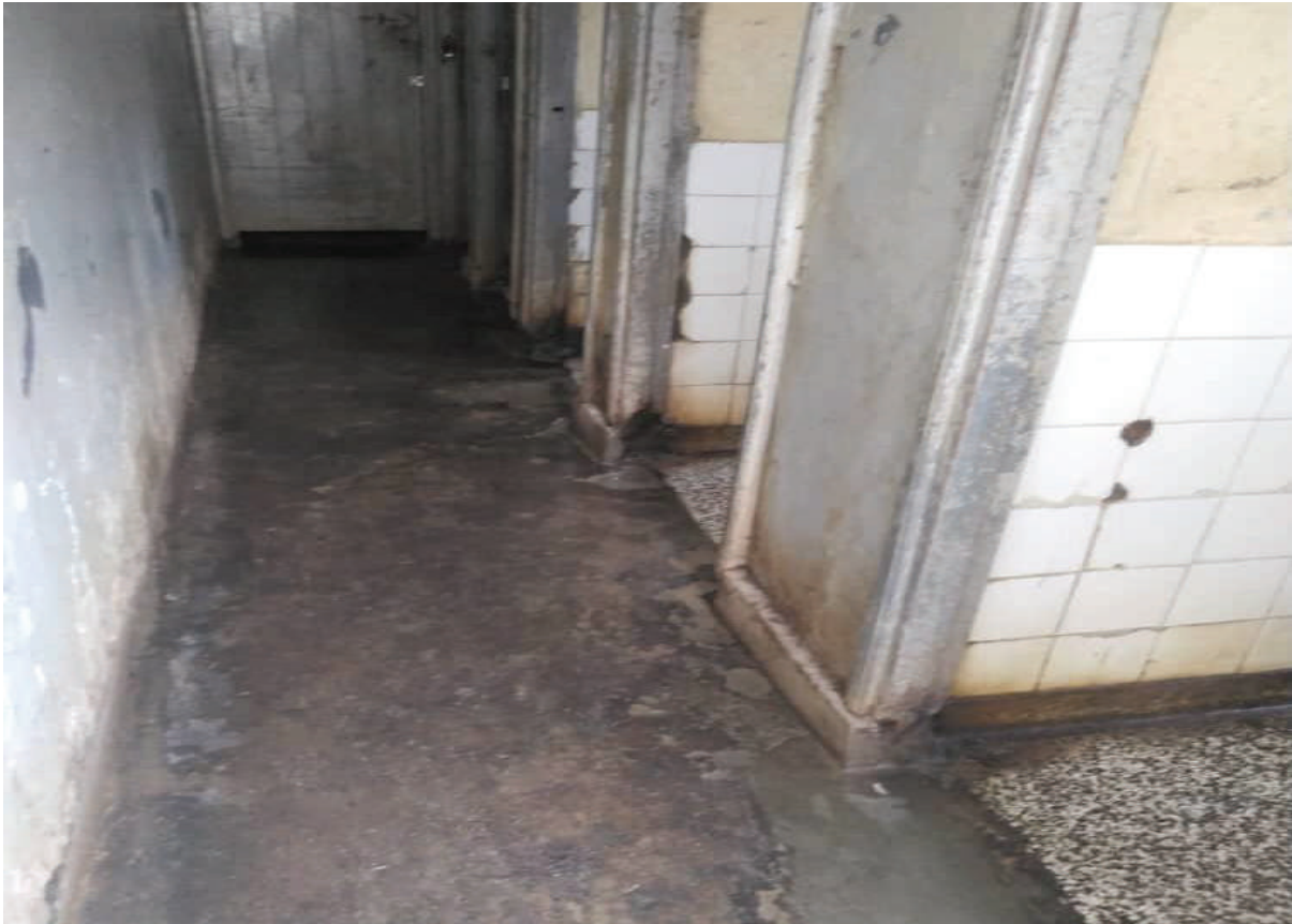
Washrooms without doors at the hospital
