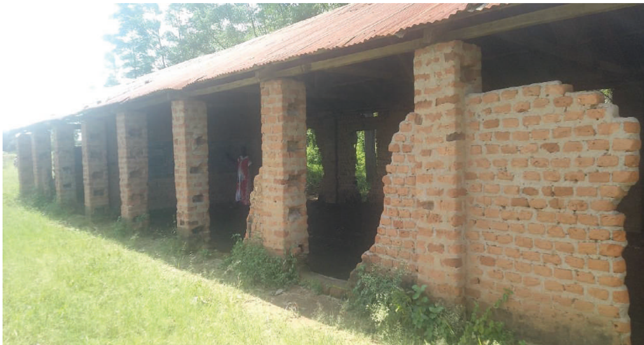
A dilapidated classroom without desks at Paipir primary school, Pader district
